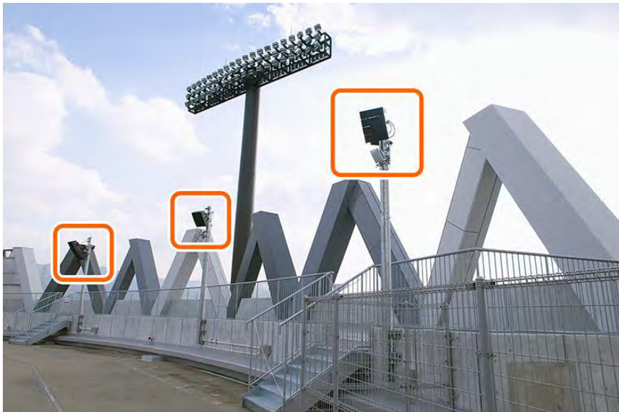
Outdoor compact array speakers distributed to face the south stands deliver uniform sound to spectator seats.
